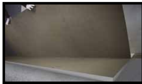
Fig.32 - Rest the slab on its long side and guide it down towards the floor.
